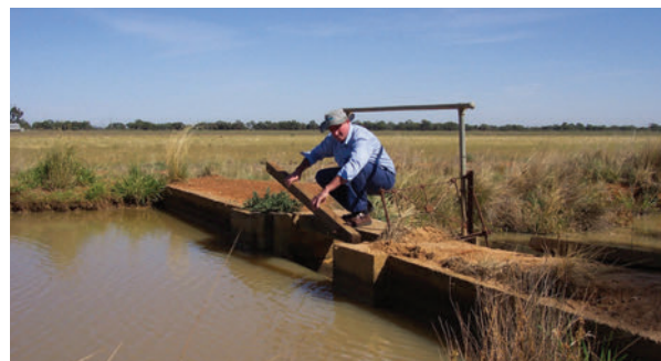
b. Manual drop bar adjustment of water level at tail regulator (Source: State of Victoria)
