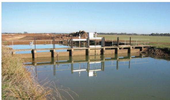
a. Overshot channel regulator, Goulburn Murray Water
