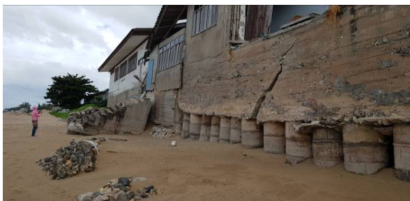
Fig. 7. Beach erosion and property damages along Ban Thung Pradu
