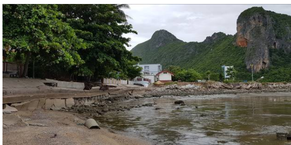
Fig. 5. Failure of shoreline protection at Ban Khlong Wan between transect 3 and 5.
