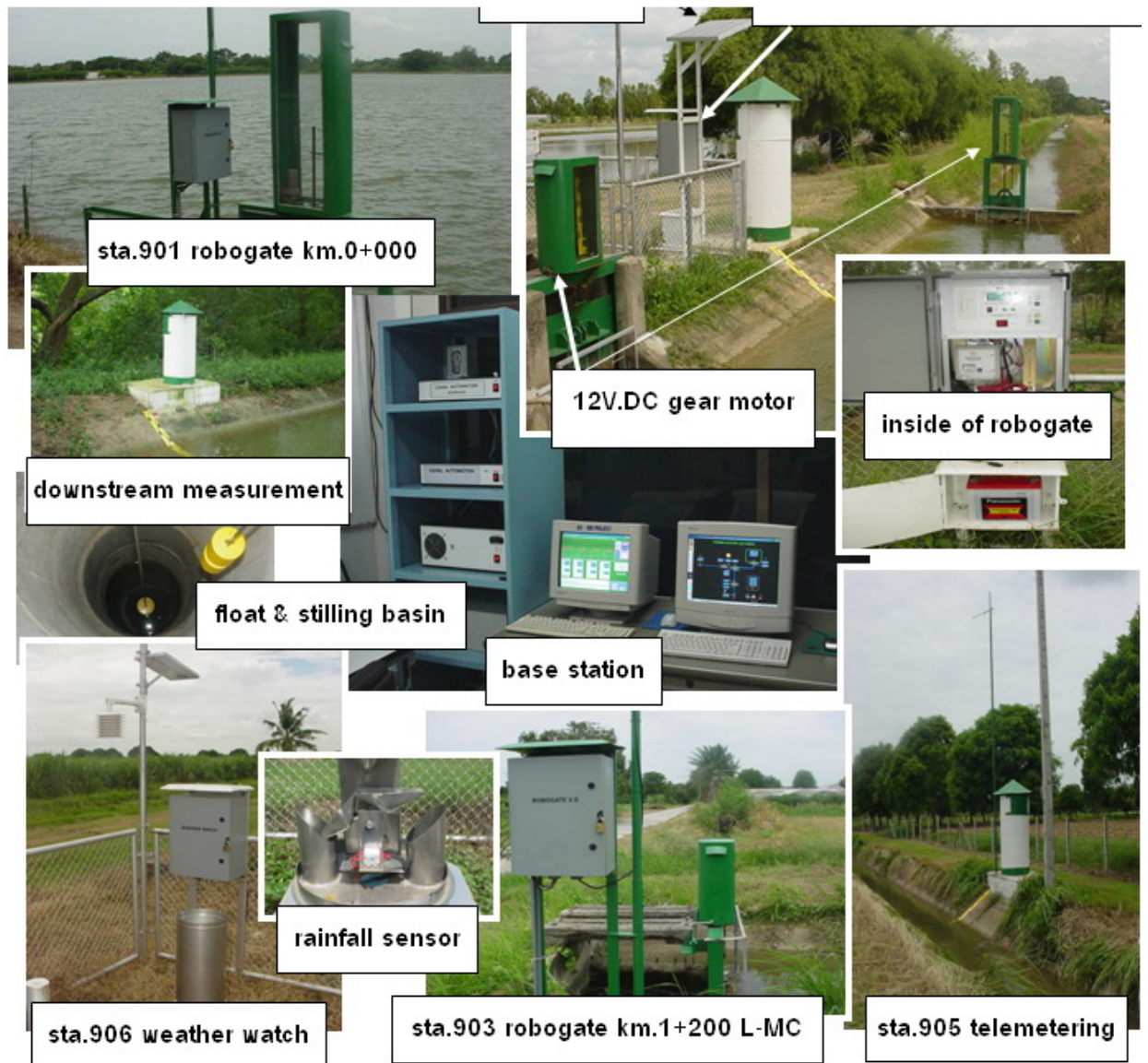
Figure 3 The installation of KPS CAS (Kamphaengsean canal automation system) devices
