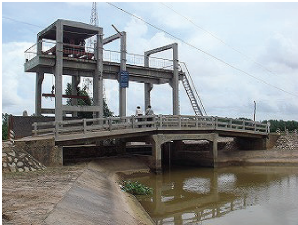
Sluice at Long Hai station
