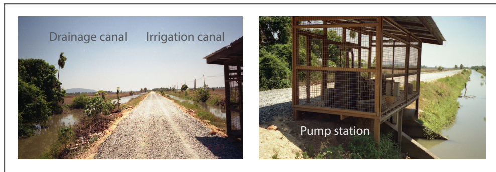
Figure 5.9 Drainage and irrigation canals and pump station for water reuse
