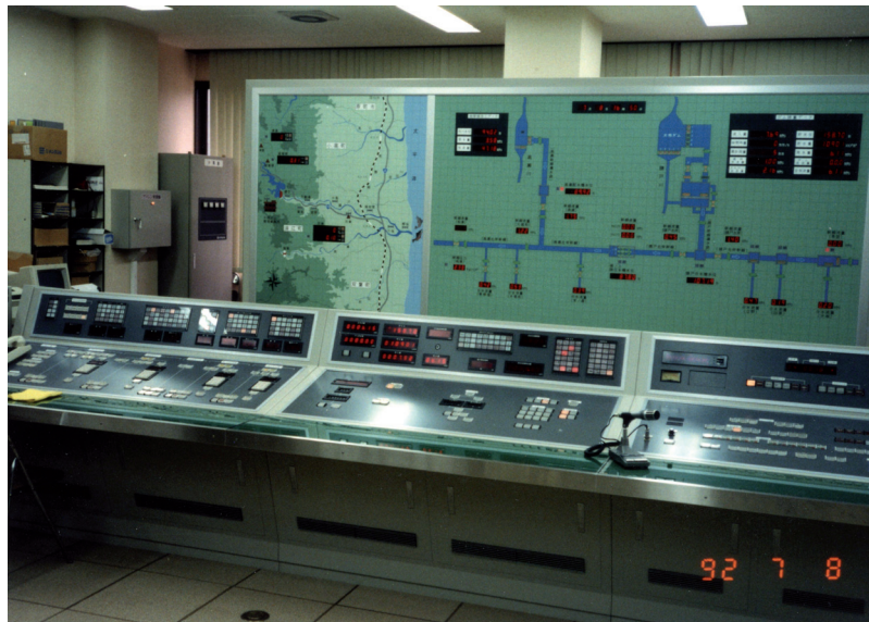
Figure 5.6 A centre for remote monitoring and control
