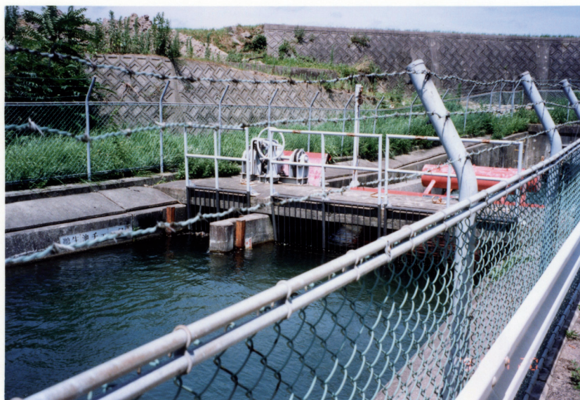
Figure 5.7 Automatic gate (control of water level upstream) accompanied by a manual gate
