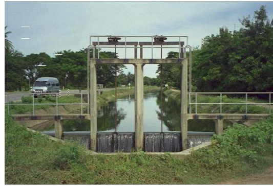
Mixed Regulator Operating in Overflow Mode (Phetchaburi O&M Project)
