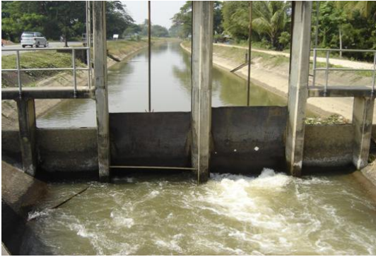
Mixed Regulator Operating in Undershot Mode (Phetchaburi O&M Project)
