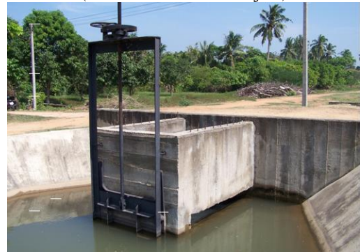
Mixed Regulator for Limited Canal Width Operating in Mixed Mode (Both Undershot and Overflow) (Phetchaburi O&M Project)
