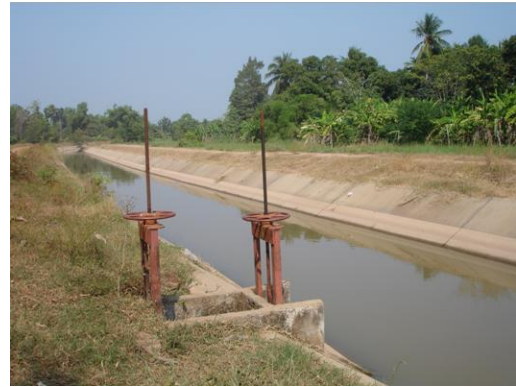
Constant Head Orifice (Borrommathad O&M Project)
